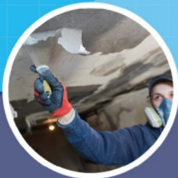
Fire & Smoke Damage Restoration
